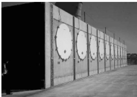
Fig.1 NUHOMS-24P Spent Fuel Horizontal Storage System at Rancho Seco Nuclear Power Station
